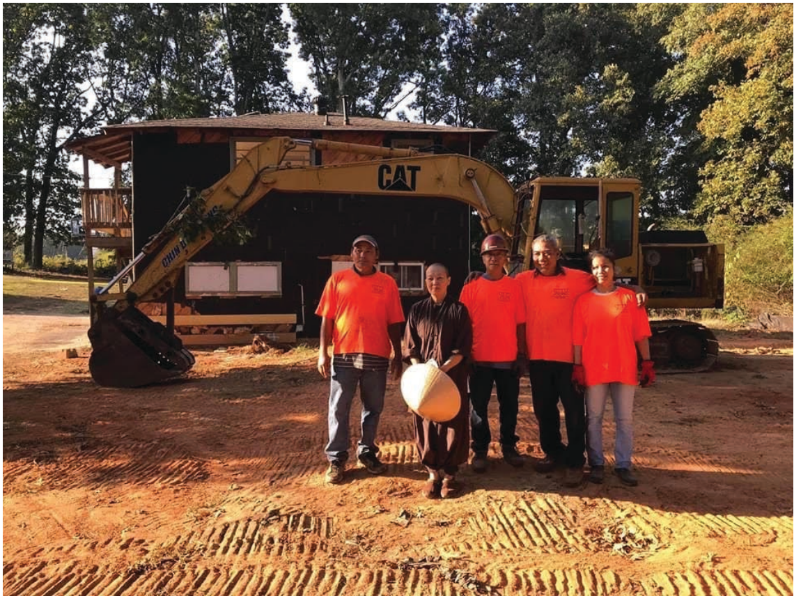
The Ven. Bhikkhunī Abbess TN Huệ Nghiêm and workers digging the foundation to build a new hall in 2020
