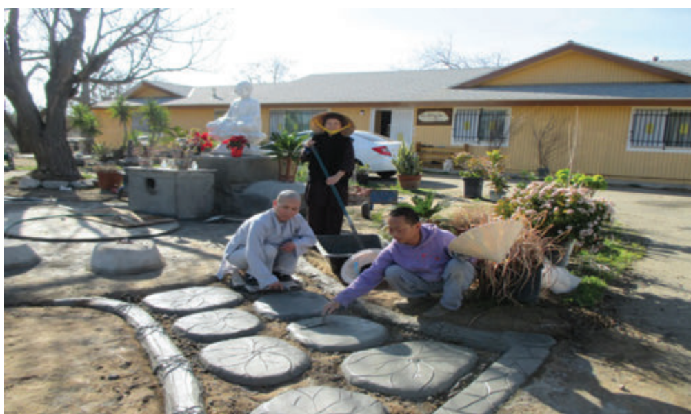
Bhikkhuni Viên Chân (mixing cement), Rev. Thiên Đức and Ven. Bhikkhuni Giới Hương making the walking path with lotus leaves
